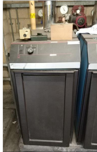
Aging gas fired boiler
