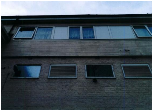
Plant room flues (below) with the site manager's flat above
