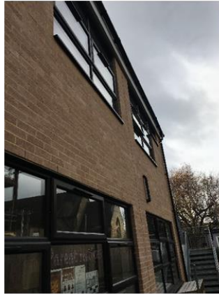
Reliance on natural ventilation worsening exposure
