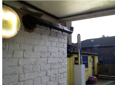
Boiler flue in foreground and main plantroom flue in background
