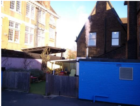
Main plant flue in playground
