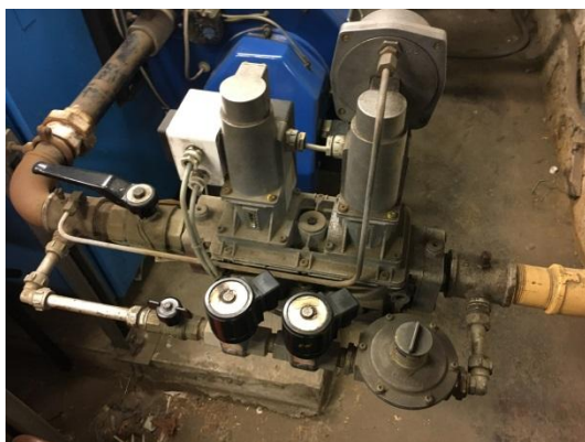
Gas powered double boiler. This is 26 years old.
