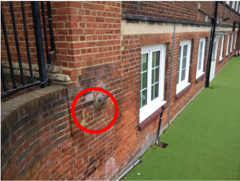
Gas boiler flue discharging at low level in KS2 playground
