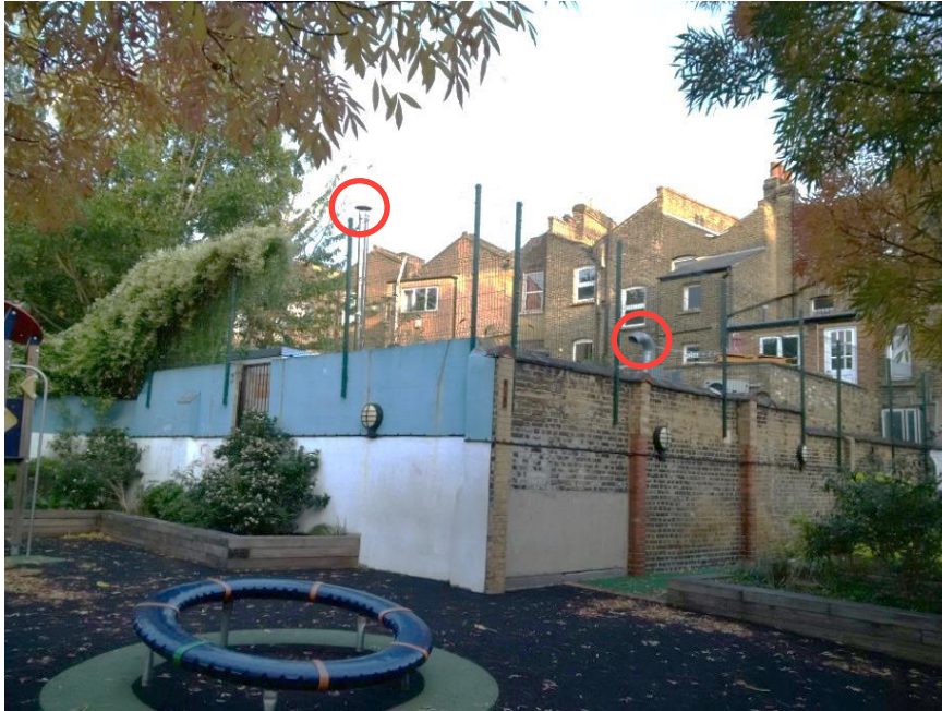
Restaurant extractor exhaust and flue from unknown source adjacent to playground
