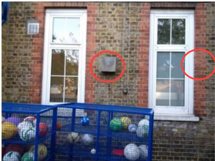
Gas boiler flue in playground by opening windows
