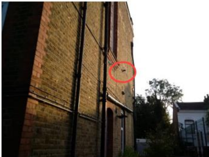
Gas boiler flue first floor level above early years playground
