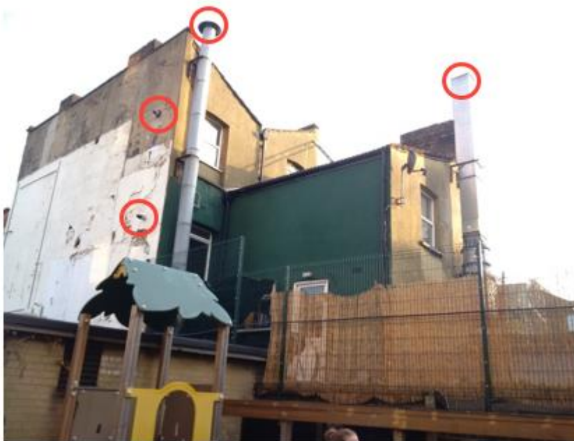
Two gas boiler flues and two restaurant extractor exhausts adjacent to early years playground
