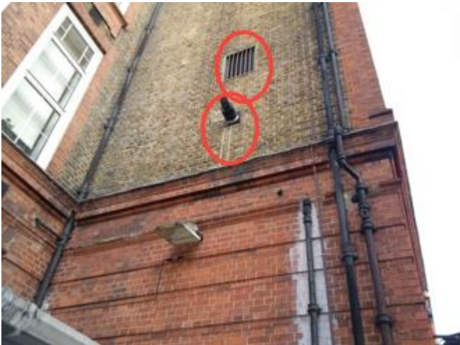
School kitchen gas fired water heater flue and kitchen extractor air intake at first floor level below opening windows and above early years playground. (Kitchen extractor vents at first floor level to right of photo)
